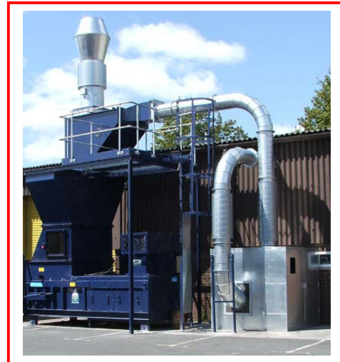
Separator serving five stitching lines
