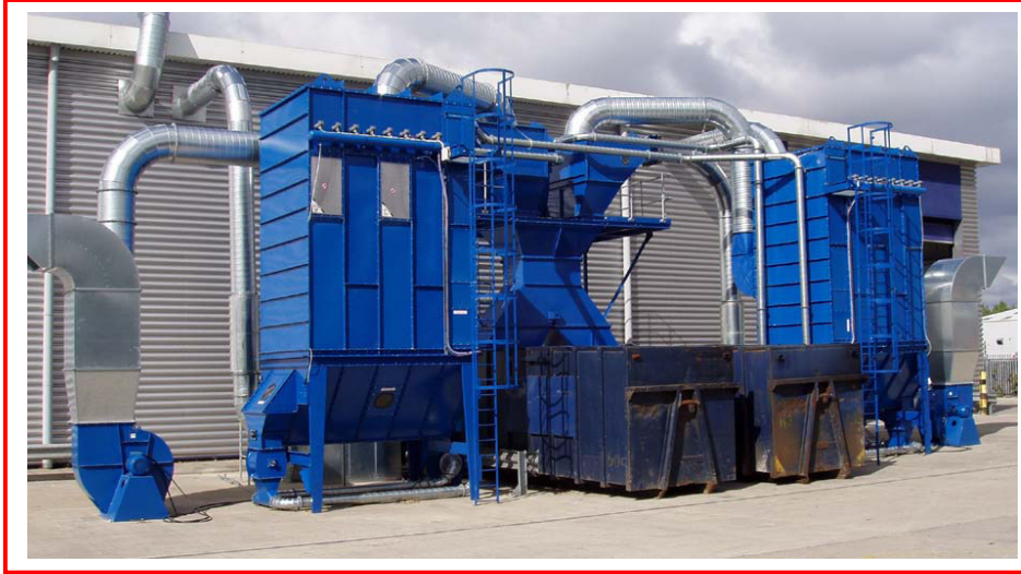
View showing a large twin compactor system at a Cardboard Box Manufacturer
