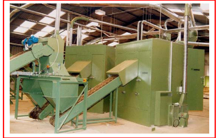
Granulators inside Acoustic Housings
