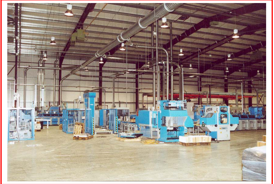
Internal Duct serving High Throughput Machinery
