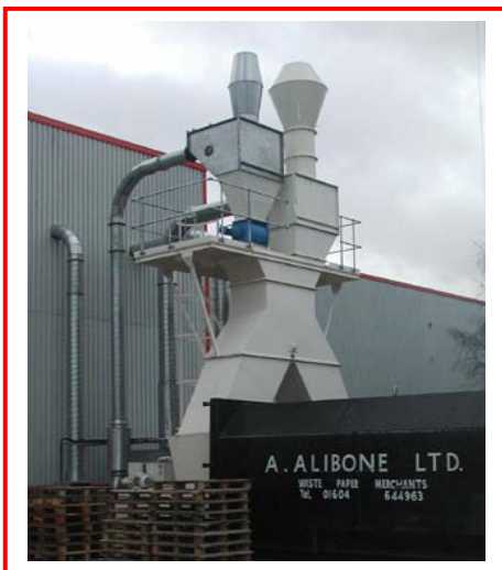
Twin Separators above Twin Compactors
