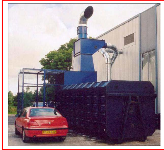
System installed at CCA - Preston
